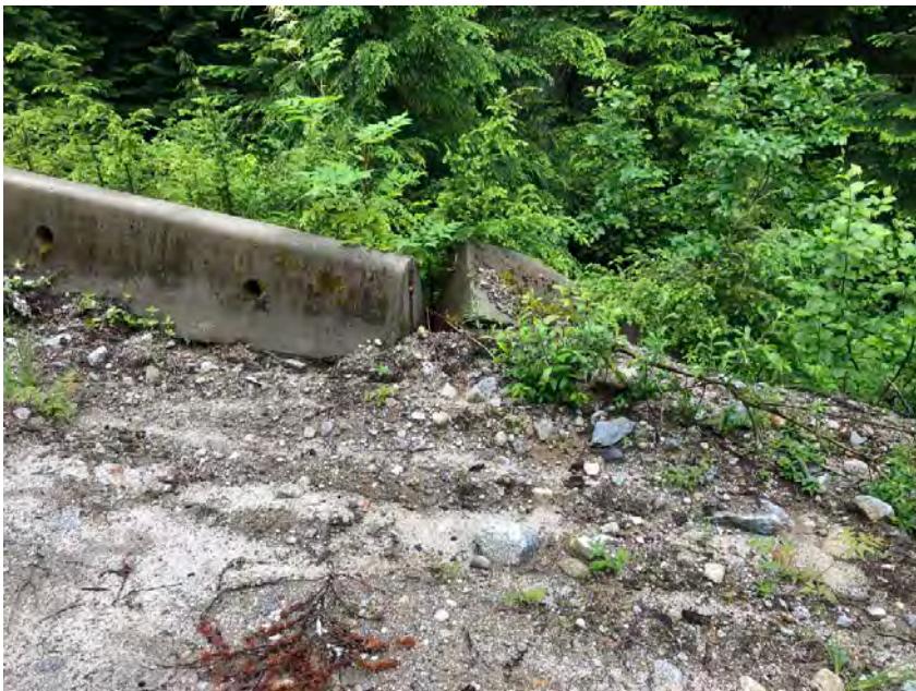
Downstream right bank bullnose not connected
